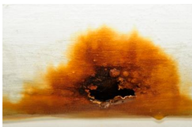
Fig. 1. Rust penetrated through an acrylic/urethane-based coating
